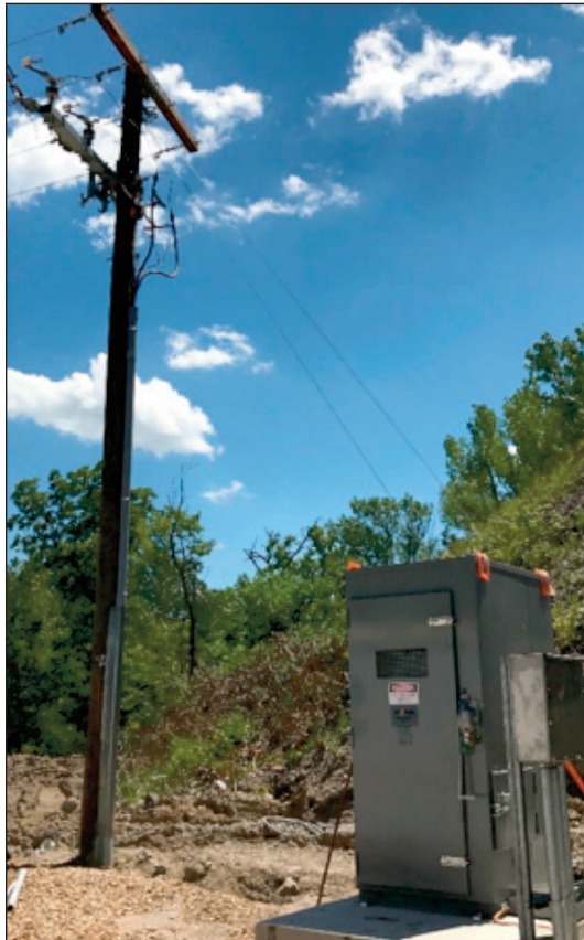
FIGURE 10: Primary Metering Pole Feed to Switch Cabinet
