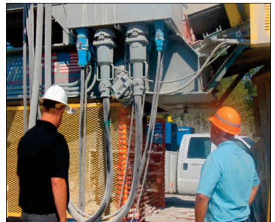
FIGURE 6: Mike Vaughn of Charleston Stone Shows Electrical Connections to Sam Adair of CMEC
