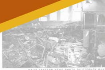
DAILY EASTERN NEWS PHOTO BY STEPHEN HAAK Damage in Blair Hall room 3114
