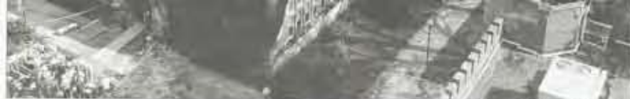
The extent of the damage to the roof of Blair Hall can be seen from the top of Old Main. The four peaks of the building will be reinforced Monday as a precaution.
